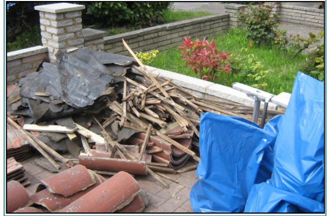
The remnants of the consumer's roof
